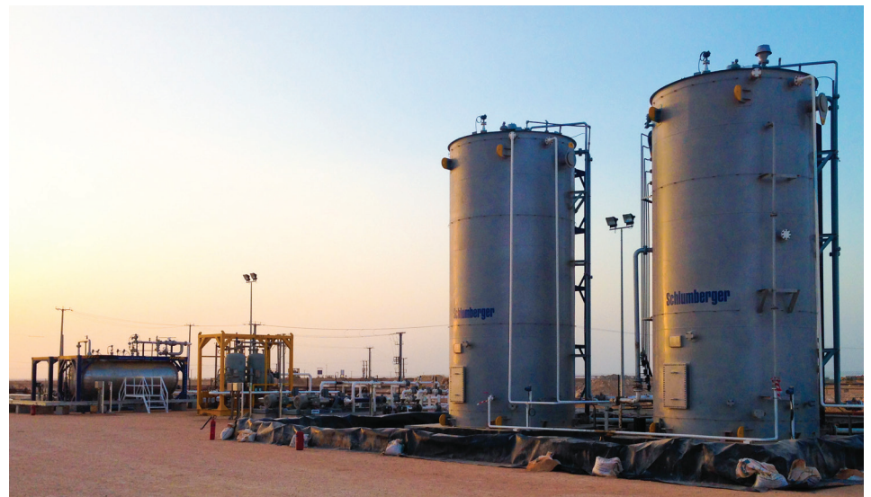
Produced water treatment system.
