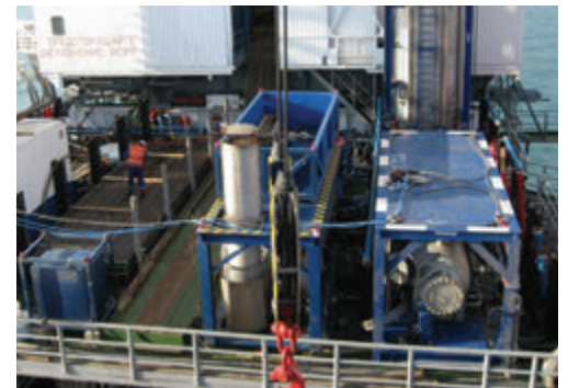
Surface well test equipment on the Lukoil Astra jackup exploration rig in the Caspian Sea.
