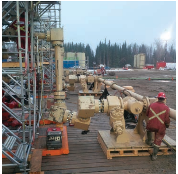
The Monoline technology uses a series of 5-in high-pressure pipe segments joined together with 90-degree elbows and swivel flanges. Shown is a nine-well pad with a single modular manifold connecting to each well, eliminating leak paths and reducing safety hazards.
