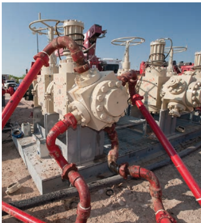
Three-leg manual and hydraulic valve isolation frac manifold
