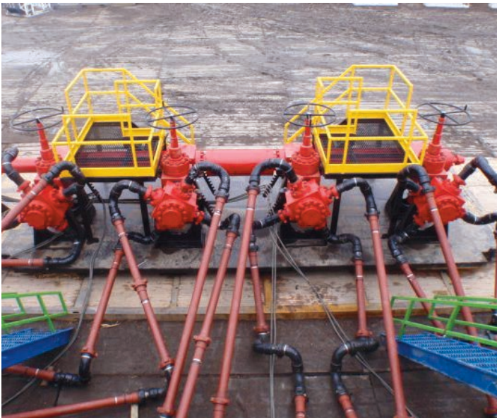
Manifolds quickly isolate wells that completed a frac cycle.
