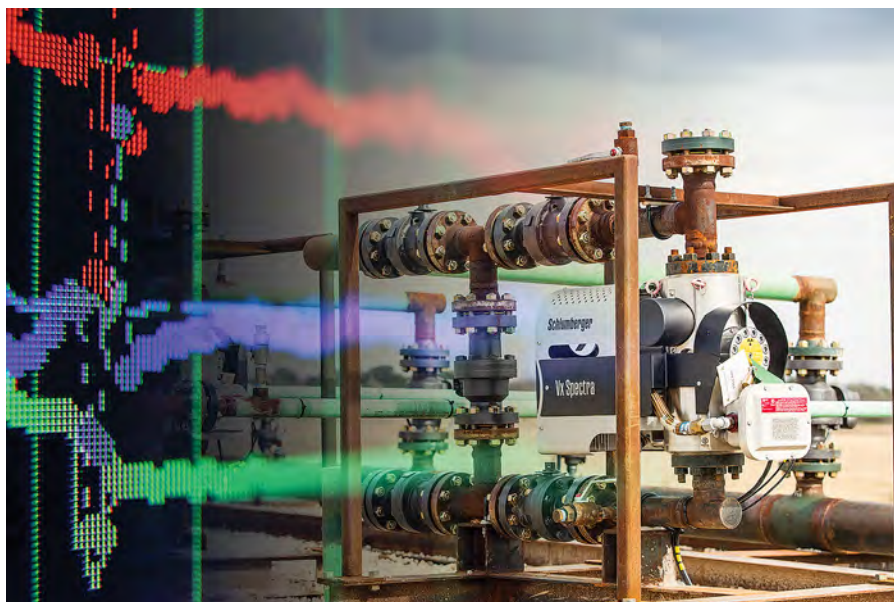
Fig. 1. Full-gamma spectroscopy analysis deployed by the surface multiphase flowmeter enables operators to determine oil, gas and water flowrates without separation.
